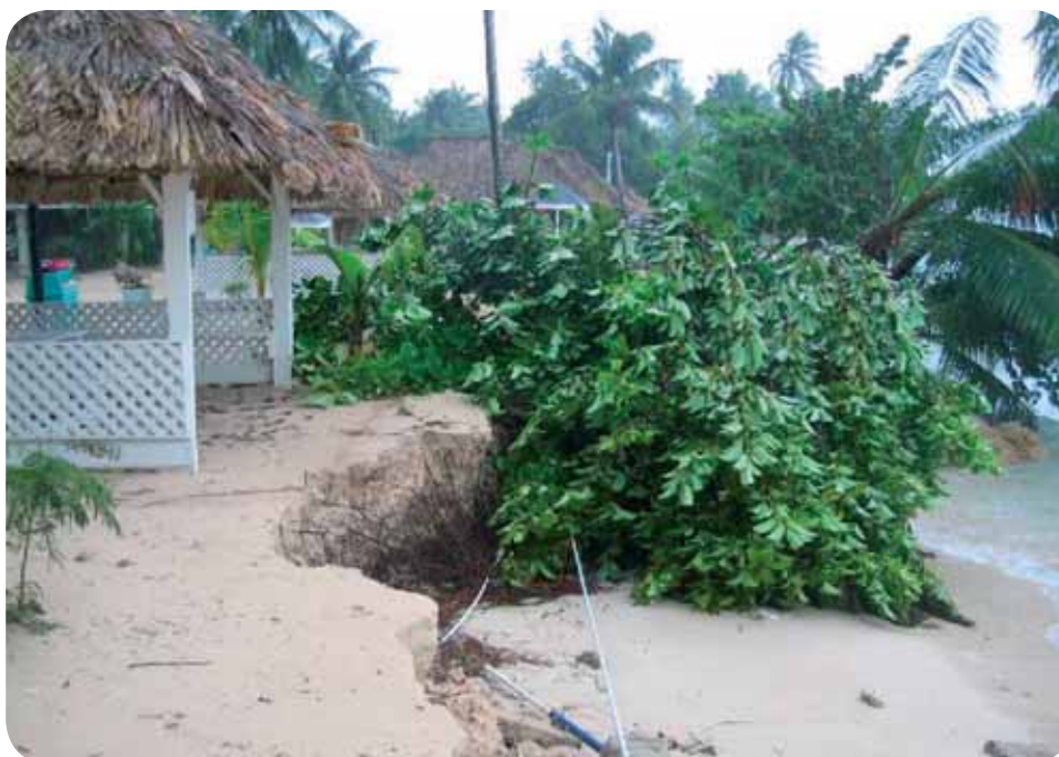
Hurricane Ivan Damage to Tourism Communications and Infrastructure, Tobago Credit: Dr Murray C Simpson
